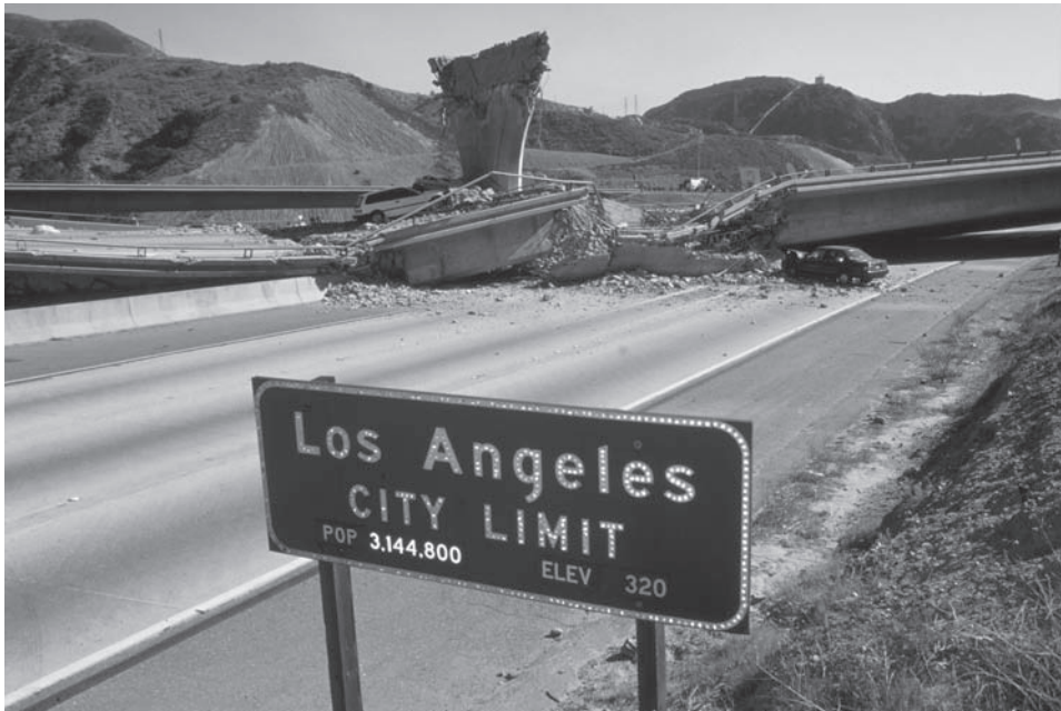
Damage to be repaired in the earthquake's aftermath.
